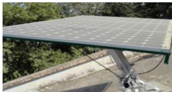
Figure 4 Designed solar tracker PV system.
